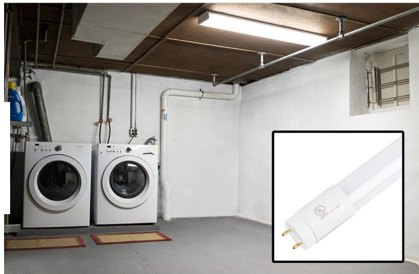
T8 LED bulb in basement tube light fixture
